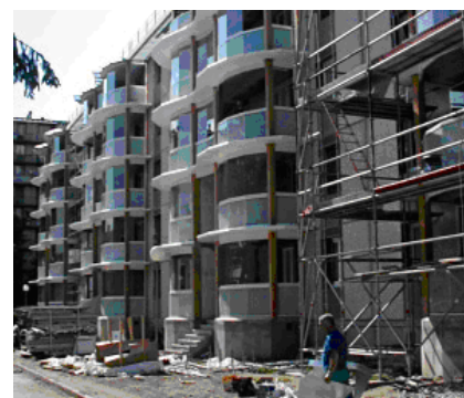
Refurbishment of social housing in Grenoble, France, uses glazed south-facing balconies to capture solar heat
